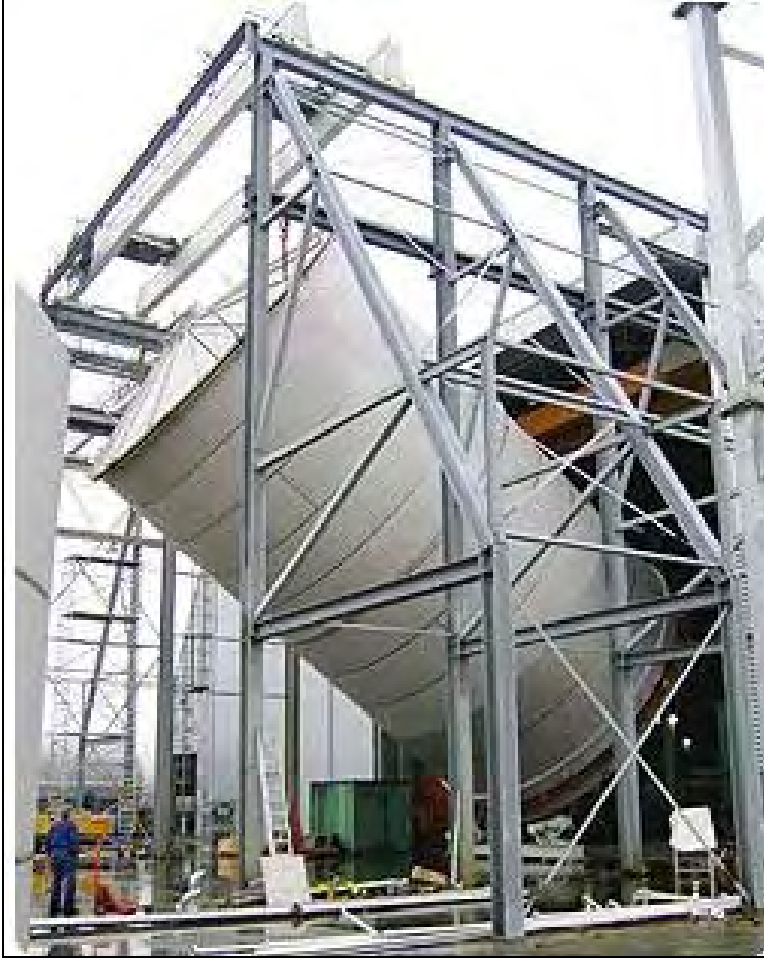
Fig. 21 LDX 2101 Tank being erected for the project Greenmills. LDX 2101 saved nearly 25% on total material used in comparison to type 304L stainless steel.
