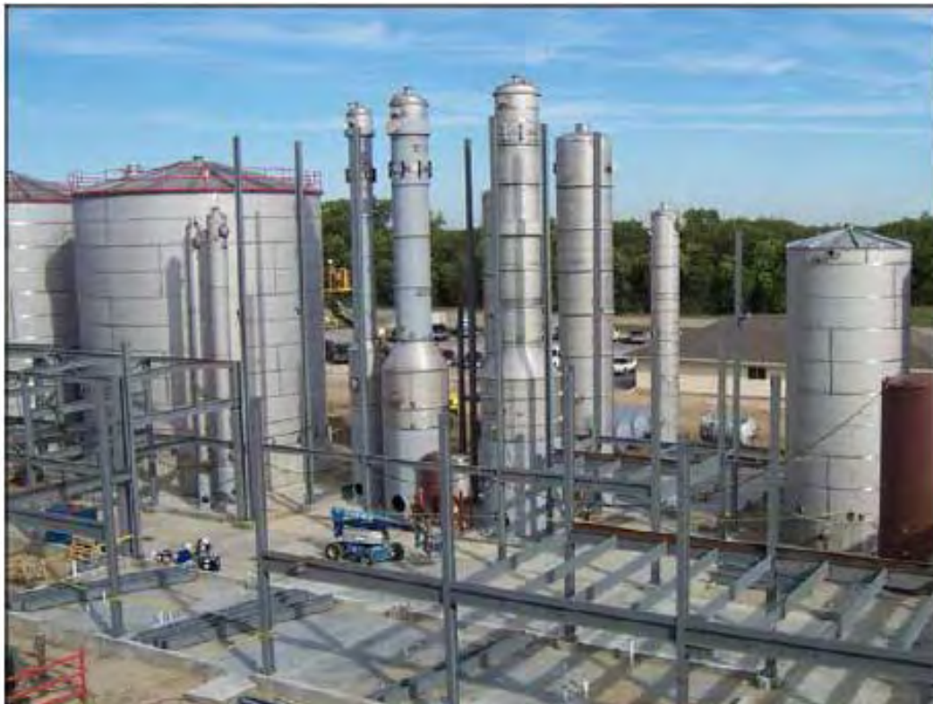
Fig. 18 Ethanol manufacturing facility during construction. Lean duplex was used for the process tanks. [6]
