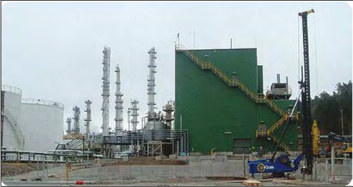
Fig. 17 Rape Seed Biodiesel facility
