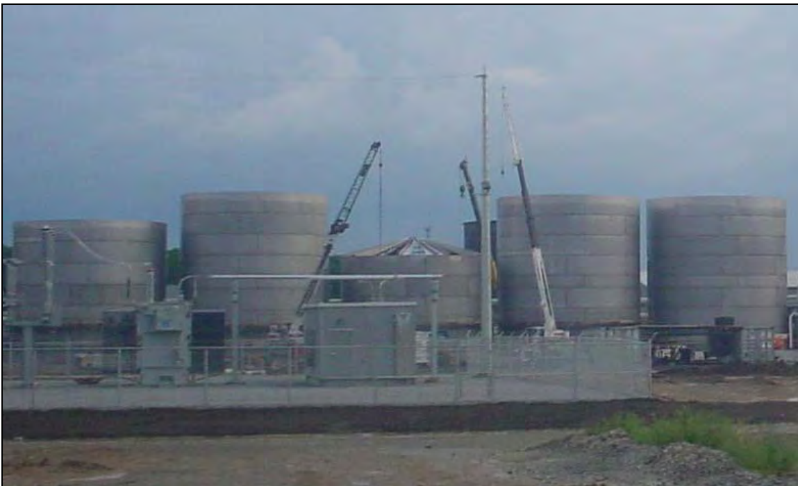
Fig. 14 View of the GO-Ethanol facility in Lima, OH during construction. All large tanks shown were constructed from the LDX 2101 lean duplex stainless
