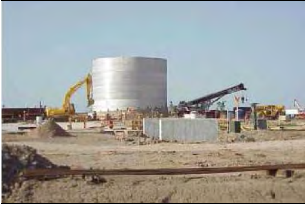
Fig. 19 Ethanol fermentation tank constructed from lean duplex stainless steel
